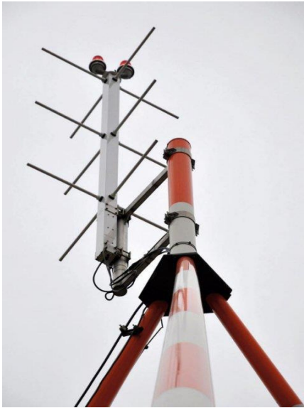
GBAS antenna at Frankfurt Airport. DFS)
